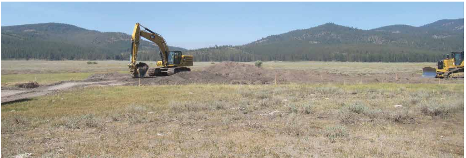
To restore Sardine Meadow, we filled parts of the channel to allow the water to spread out and meander across the surface. Photo: Beth Christman
