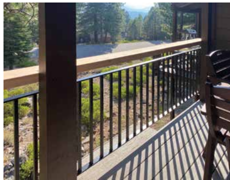
A demonstration deck was installed at 6059 Rocky Point Circle and you can get an idea on how it will look.
